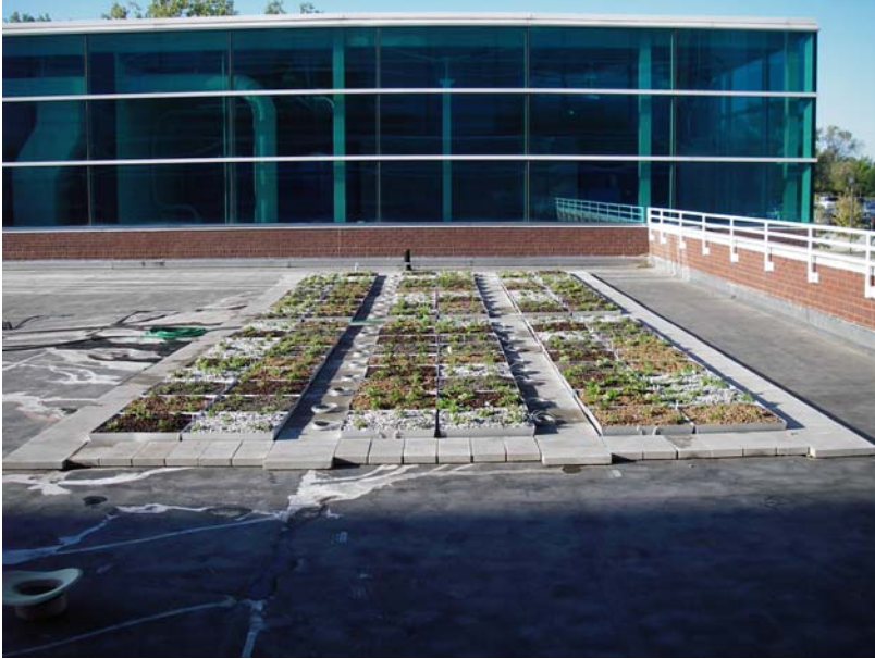
Figure 1. Green roof project on the roof of the Southern Illinois University Edwardsville Engineering Building.
