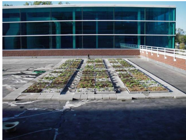
Figure 2: Picture of Phase I of the project layout, which was installed in a completely randomized design on the roof of the Engineering Building on the SIUE Campus on September 20, 2005.
