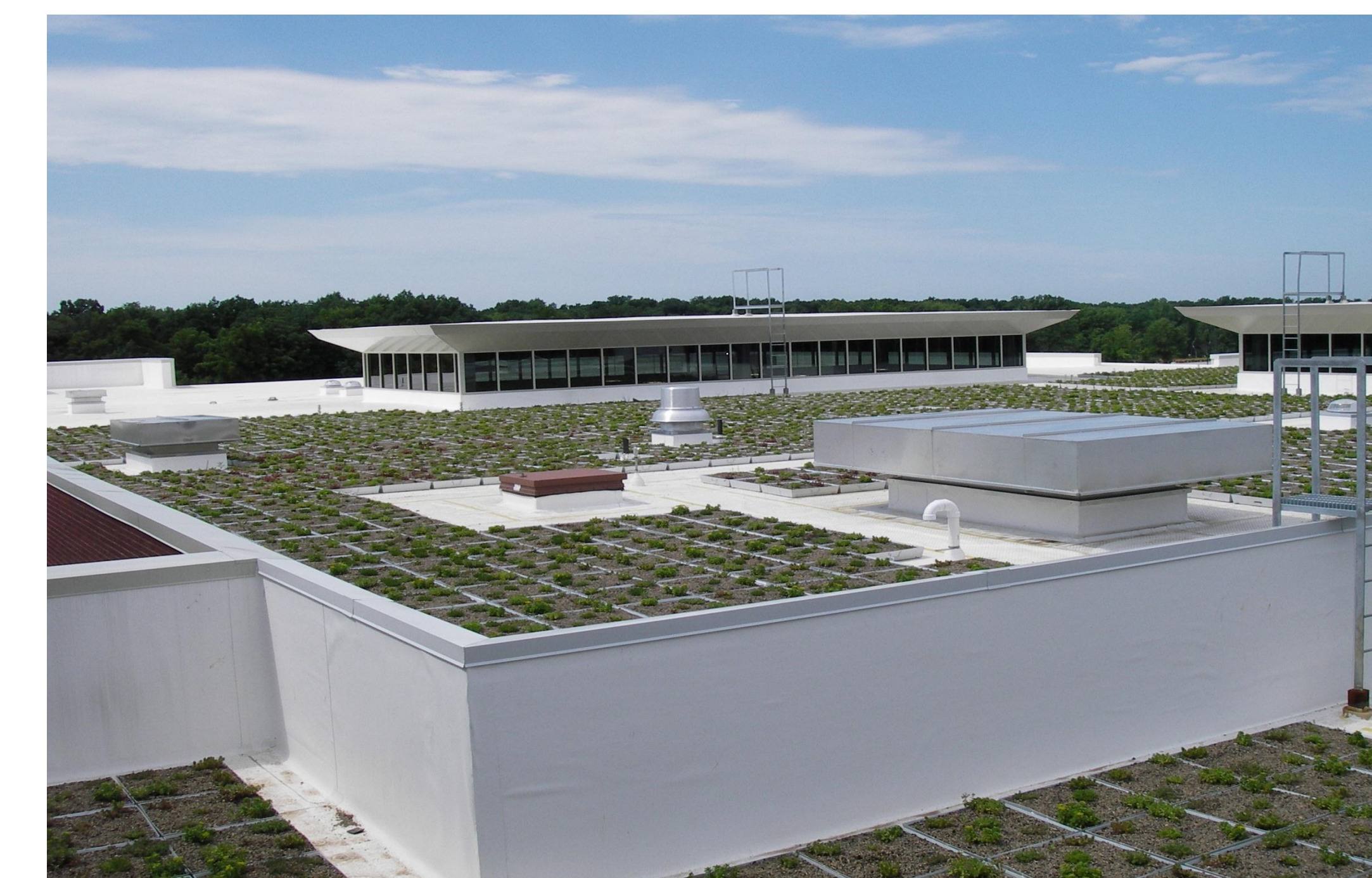
Figure 5: Green roof on the Student Success Center at Southern Illinois University Edwardsville. Established using plug plants in Green Roof Blocks™.
