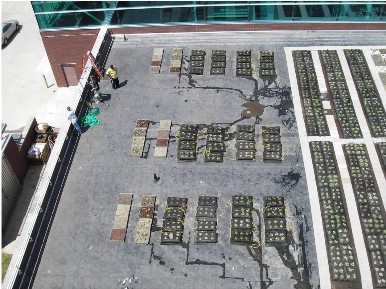
Figure 1. Green Paks™ and Green Roof Blocks™ on the SIUE Engineering Building roof after installation on May 23, 2007.
